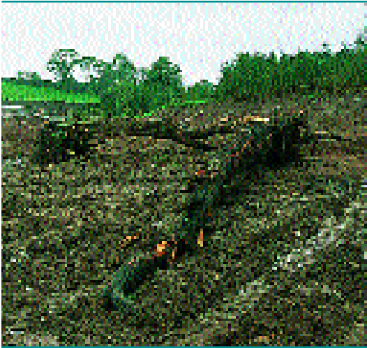
Road improvements with loss of mature trees and hedges
