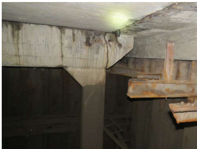
Figure 2 – Portal frame to be repaired
